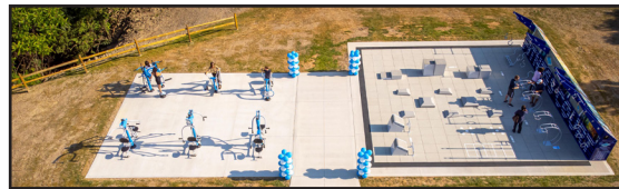
The Public Works Department cleared, leveled and poured concrete to the required specifications prior to install.
